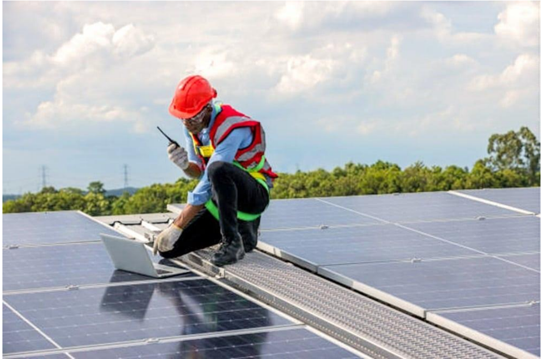
Picture 2: Up to 1 week to complete the commissioning with DNSPs
